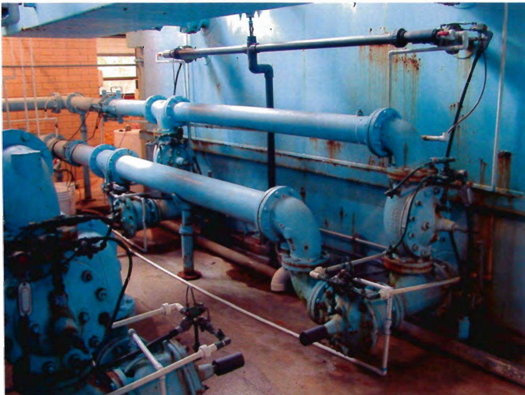
FIGURE 5.3.7 COOPER CREEK WTP FILTER UNIT & PIPING
