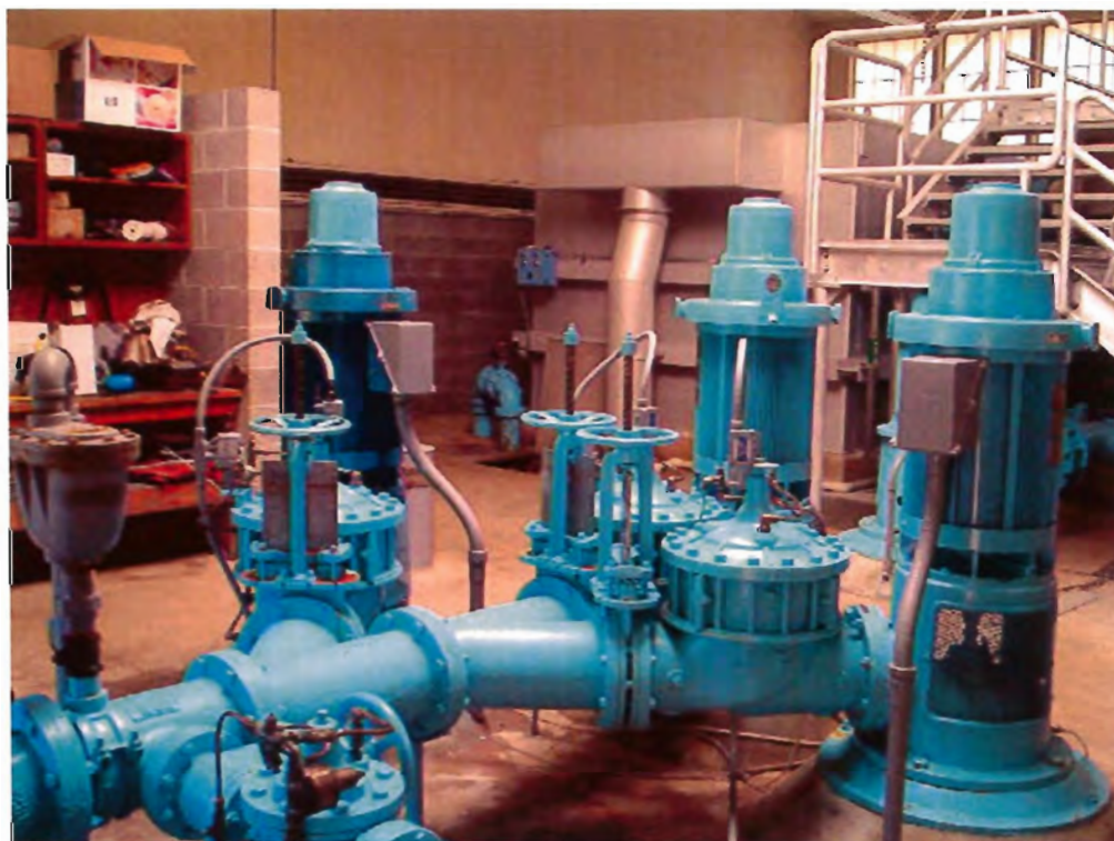
FIGURE 5.3.3 NONPAREIL WTP TREATED WATER PUMPS
