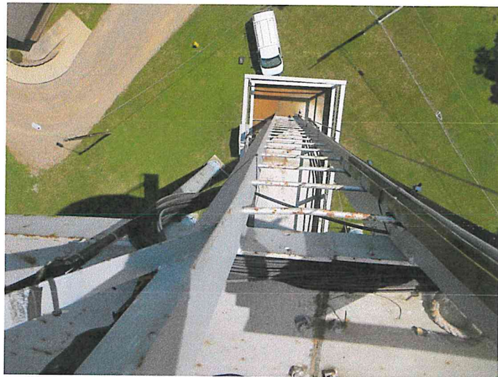
14) The ladder from the platform to the balcony is in good condition. The cable-type fall prevention device is undersized.
