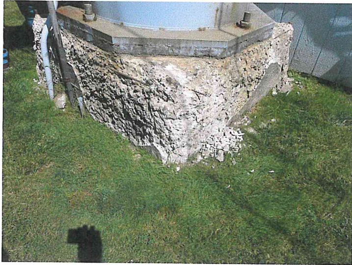
1) Typical leg foundation concrete is in poor condition.
