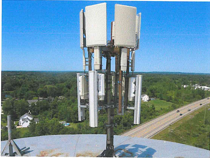
22) There is an antenna mount on the roof.
