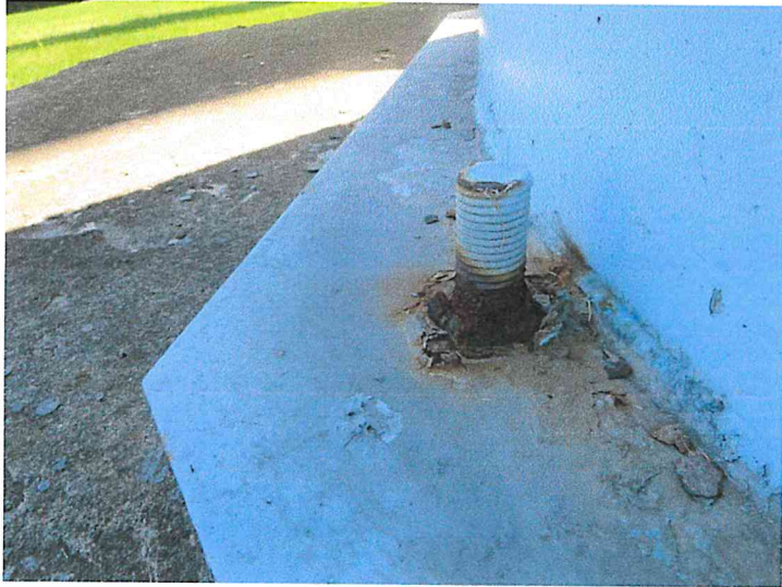
4) Anchor bolt nut completely corroded.
