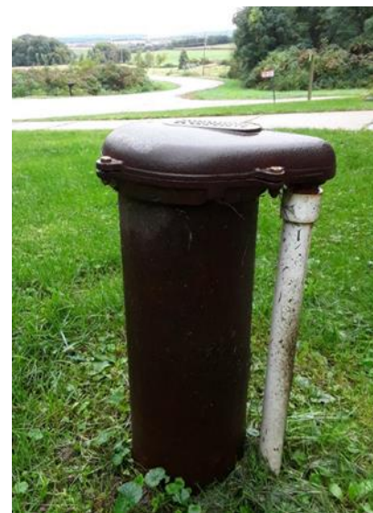
A private well used to supply water to rural residential home.
