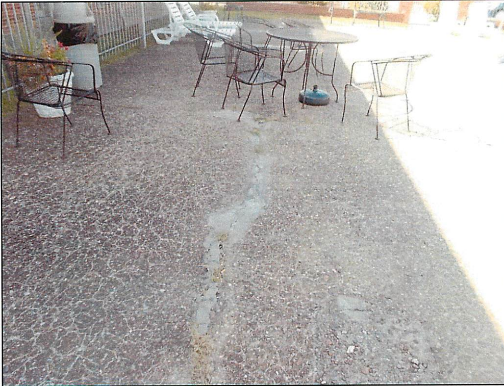
Cracked pavement in the pool area.
