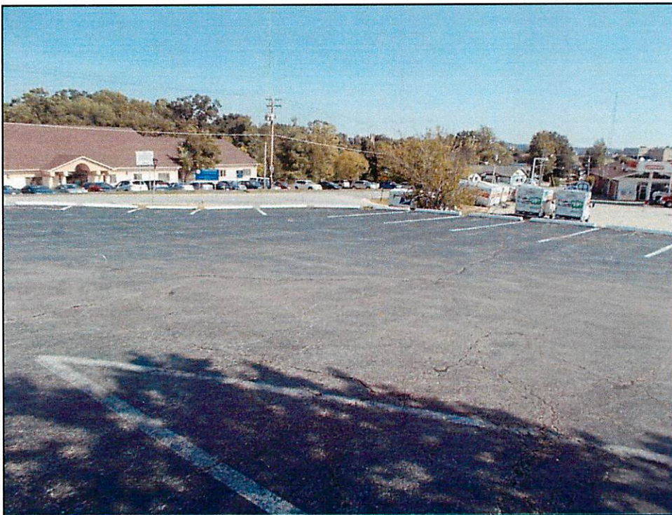
Cracked pavement in parking area.
