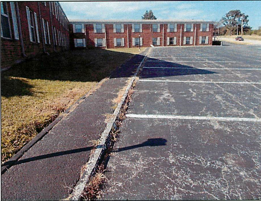
Cracked pavement showing deterioration of parking lot.
