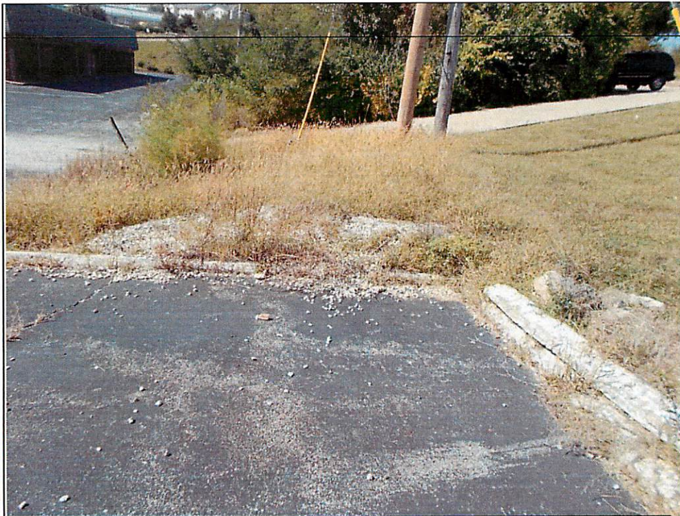
Deteriorated curbing and gutter.
