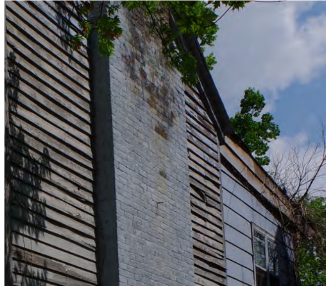
The siding on 105 Jackson is deteriorated.
