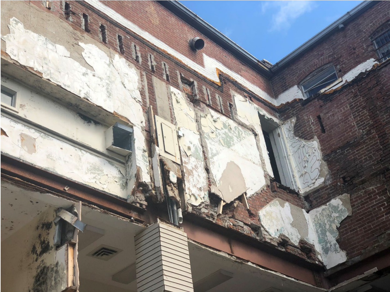
Pictures of Building for tuckpointing and mortar work areas of most concern:
