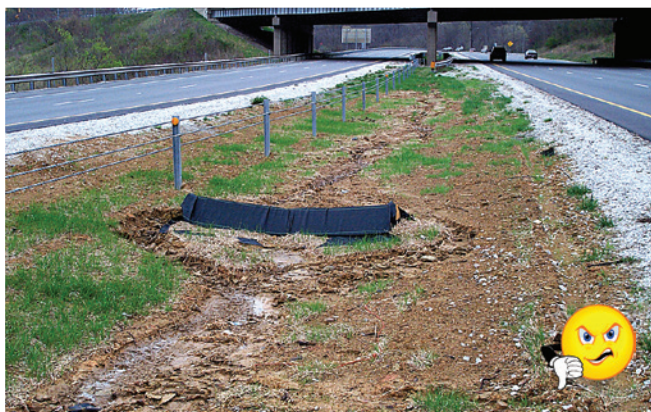
Poor application of commercial check dam product (note erosion around edges). The check dam needs to be longer (tied into the banks), and more check dams are needed, at the correct spacing for channel slope.
