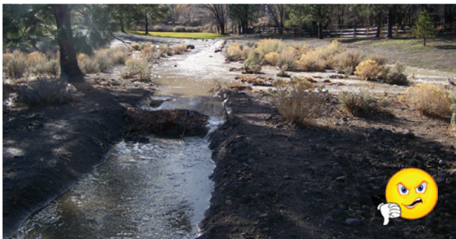
Poor protection of a waterway with fiber rolls being left in the middle of an active channel.
