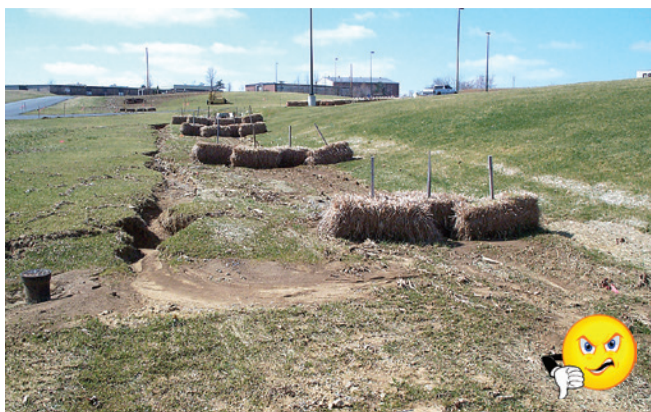
Poor check dam installation. Straw bales should not be used as check dams due to rotting, installation difficulties, and high failure rates. This check dam application should be longer for the volume of runoff and the BMPs should be spaced properly to stop/slow the water.
