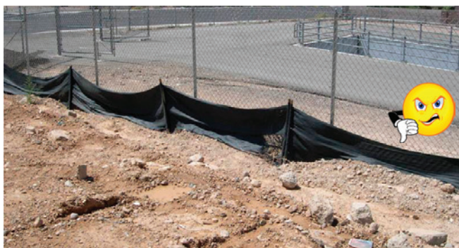
Very poor silt fence maintenance. Fences and other sediment control BMPs must be inspected and repaired weekly.
