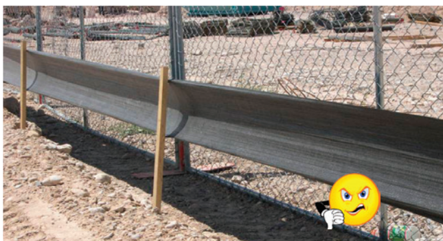
Incorrect installation. The base of silt fences must be trenched into the soil. Incorrect BMP installations cost developers money, are ineffective, and can lead to permit violations and jobsite closures.
