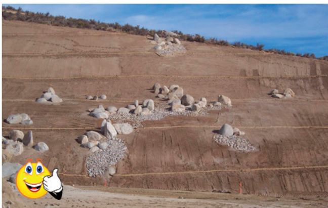
Excellent % slope reduction and soil roughness with a combination of techniques. However, fiber rolls are spaced too far apart (more than 20').
