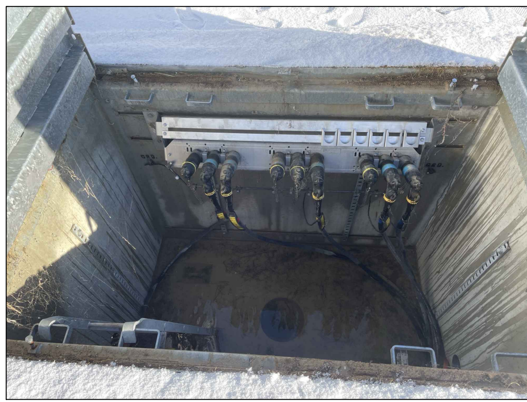
(E) VAULT CV58470
