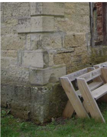
Missing quoins (bottom three stones at corner in this image). (5/20/2014)
