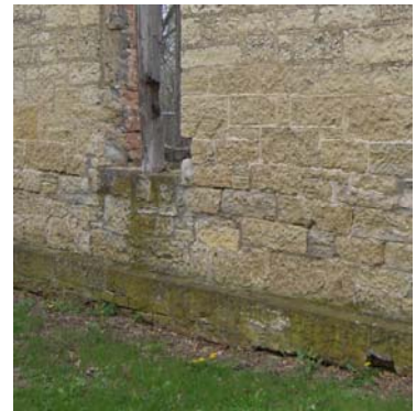
Cracks in bottom stones (at grade) (5/20/2014)
