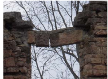
Second floor window lintel facing stone held in place with coating/cap (5/20/2014)
