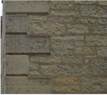
Quoins at corner (left) and square beaded joint in facing stone (right). (5/20/2014)
