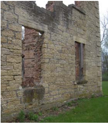
Biological growth on ruins (seen at window sills and top of wall in this image). (5/20/2014)
