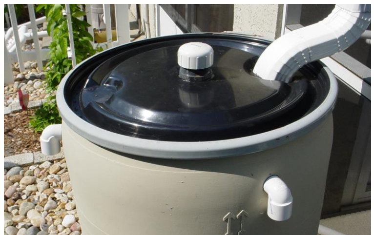
Rain barrel attached to home downspout
