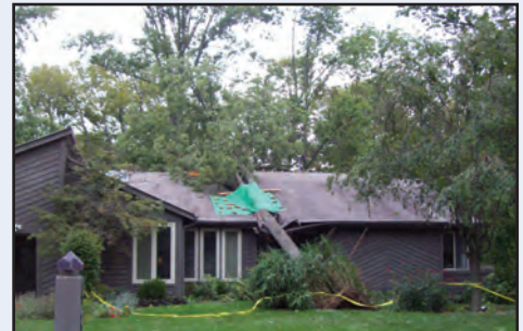
Major damage was done to this house in the Peppermill Farms neighborhood.
