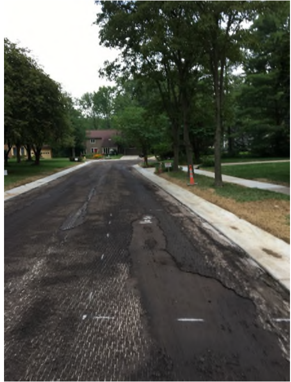
Milled road w/ area marked for full depth repair
